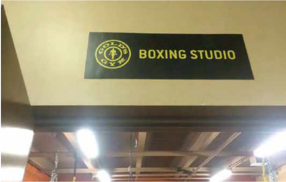
Photo 09 - Lead-Positive Ceiling (Boxing Studio)
