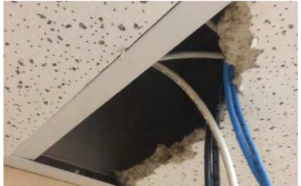
Photo 08 - Drop Ceiling Tile (Sample L1)
