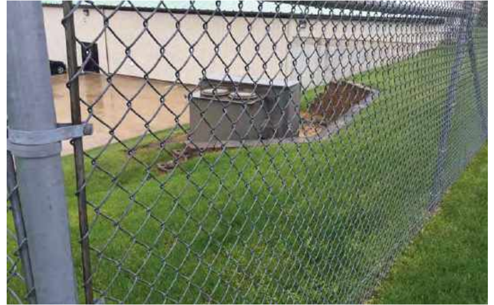
Target Property 1 - Photo 02 - Pad-Mounted Transformer
