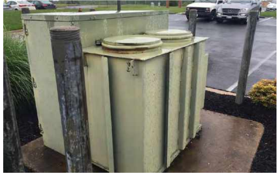
Target Property 2 - Photo 04 - Pad-Mounted Transformer
