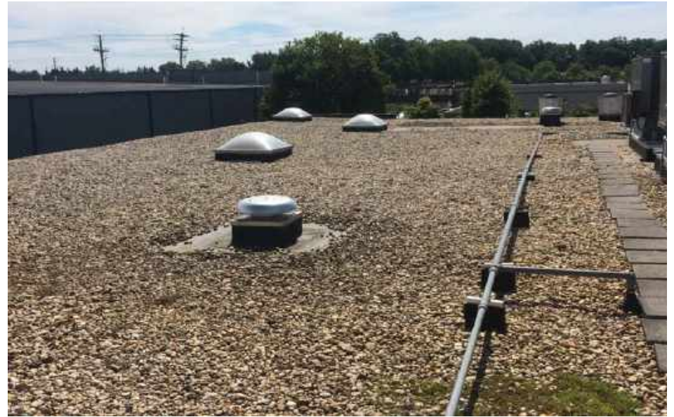
Photo 06 - HVAC System on Roof (Samples X1 and X2)
