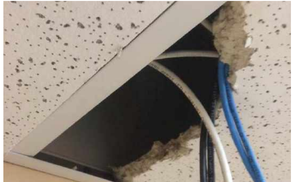
Photo 08 - Drop Ceiling Tile (Sample L1)
