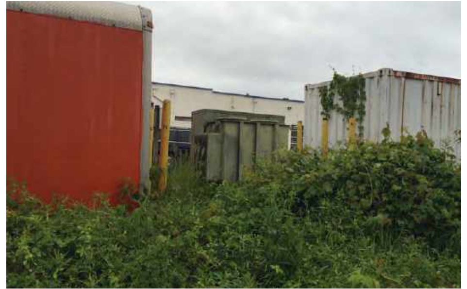
Target Property 3 - Photo 05 - Pad-Mounted Transformer and Storage Containers
