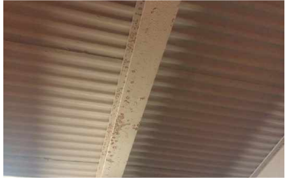
Photo 10 - Lead-Positive Ceiling (Boxing Studio)
