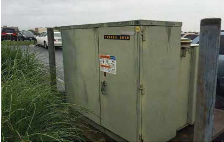
Target Property 2 - Photo 03 - Pad-Mounted Transformer
