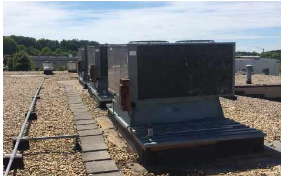
Photo 04 - HVAC System on Roof (Samples X1 and X2)
