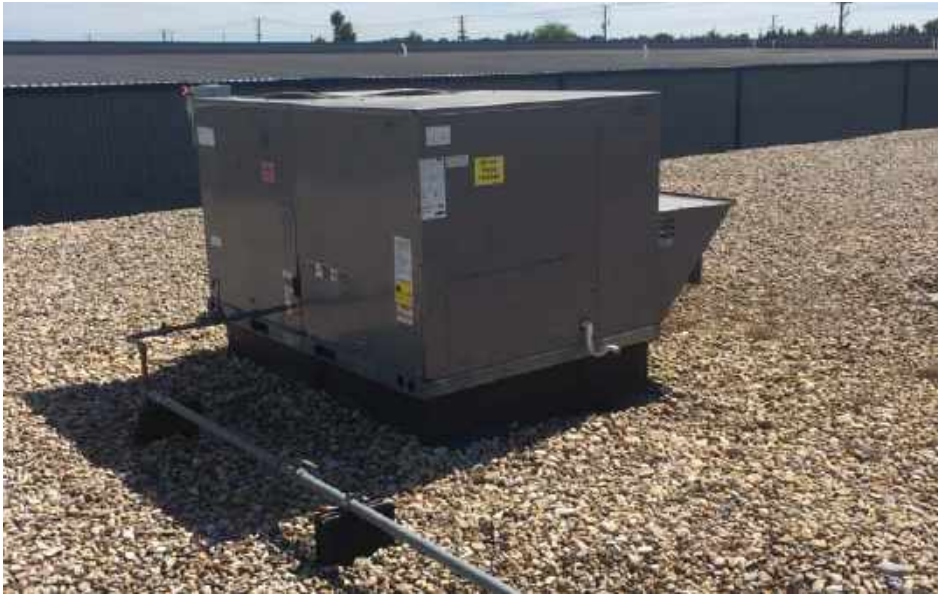
Photo 05 - HVAC System on Roof (Samples X1 and X2)
